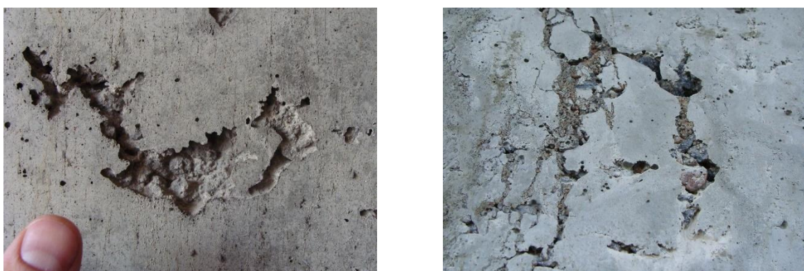
Fig.2. Macro-sized voids on the concrete surface
