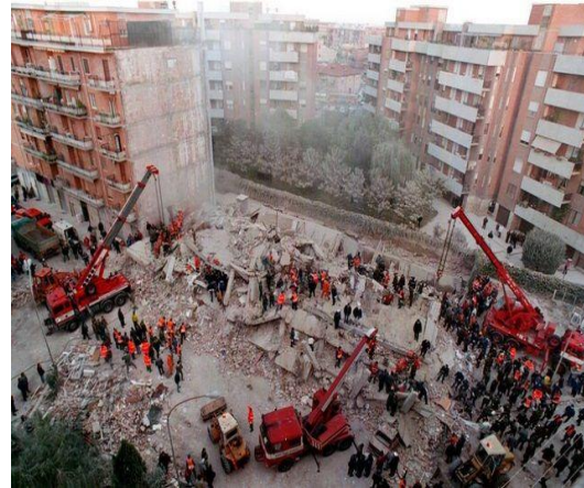
Fig. 5. A ruined house in Foja
