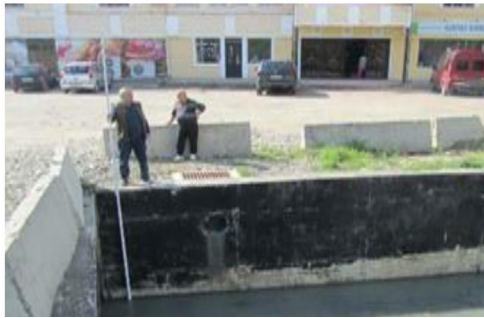
Fig. 5. Is presented on April 27, 2023, at the moment of measuring the water level of the left bank of the river Oghaskura and at the reinforced concrete bridge connecting the right and left banks of Oghaskura.
