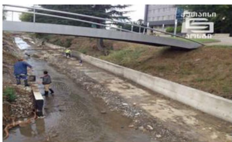
Fig. 2. In Kutaisi, the reconstruction of the river Oghaskura bed and the bridges on it.
