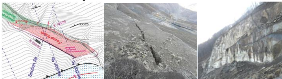
Figure 2. The topographic plan, top view and a section of remained rock block - "Southern Cliff".
