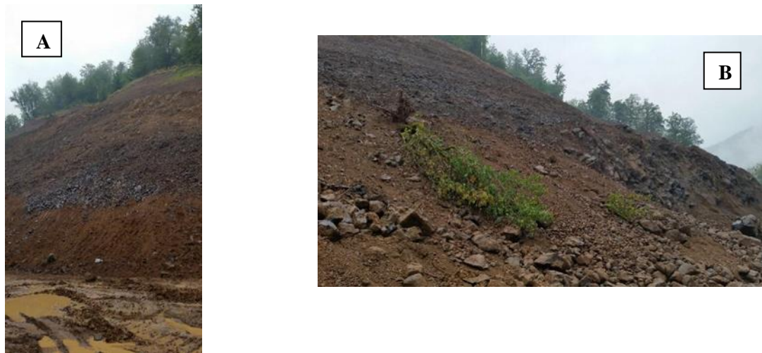
Figure 6. Active landslide processes at 17–19 km of the Lankaran–Lerik highway (photo 07.03.2021)
