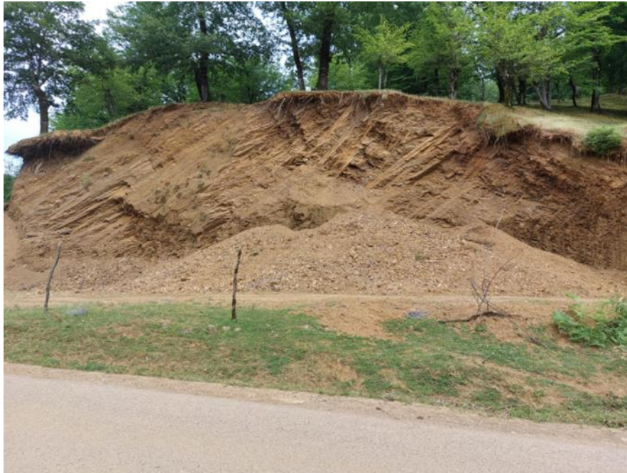
Figure 11. Landslide on the Degedi–Pelikesh road, Astara district (photo May 28, 2023)
