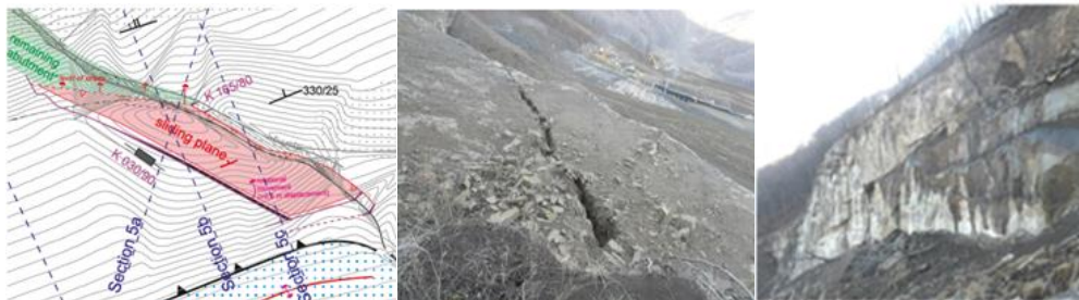
Figure 2. The topographic plan, top view and a section of remained rock block - "Southern Cliff".
