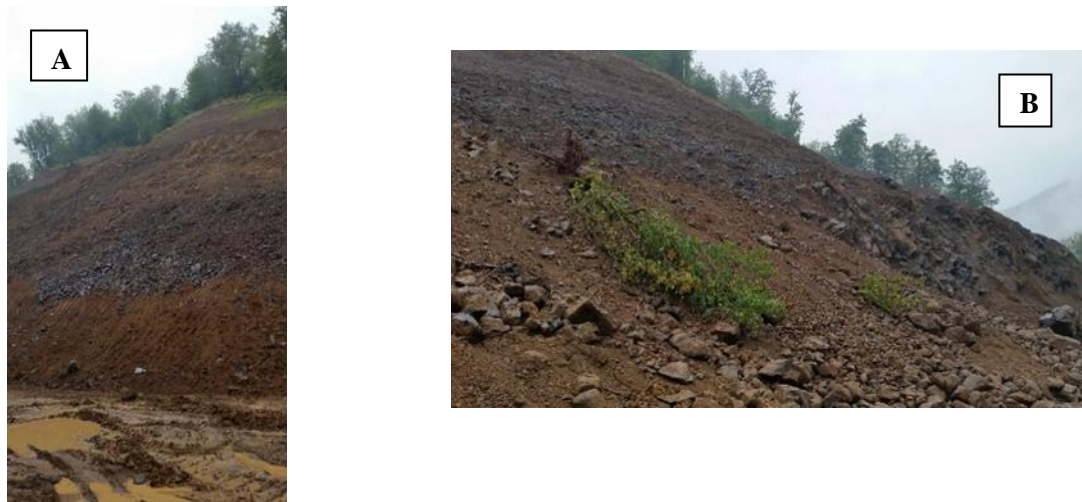
Figure 1. Active landslide processes at 17–19 km of the Lankaran–Lerik highway (photo 07.03.2021)
