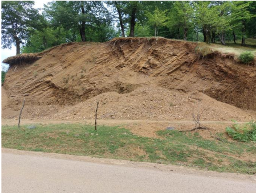
Figure 6. Landslide on the Degedi–Pelikesh road, Astara district (photo May 28, 2023)
